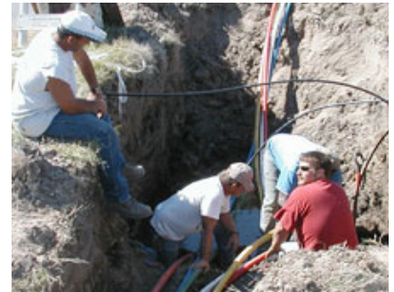
Actual site of disaster with unsafe trenching operations (Photo from www.osha.gov ).
